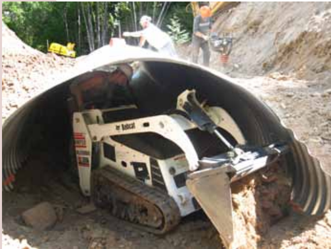
Placing a small aquatic organism passage culvert on the Lolo NF, September 2006. Photo by Traci Sylte
